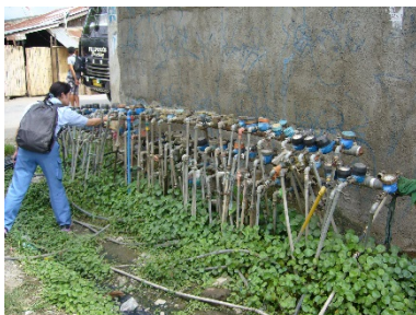
82 water meters branched Stub-Out
