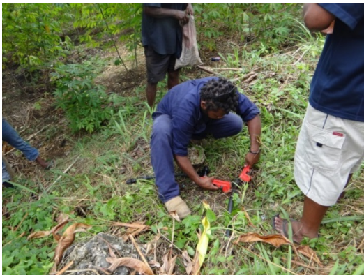
Disconnecting illegal connection
